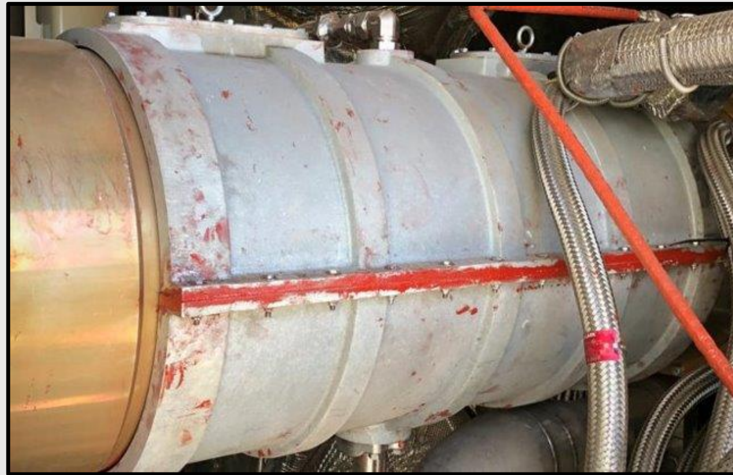
Coupling Covers with RTV sealant
