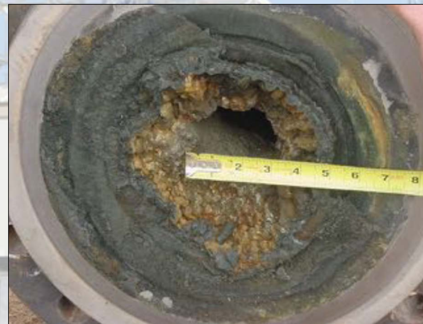
Scaling Deposition of the Current Pipeline
